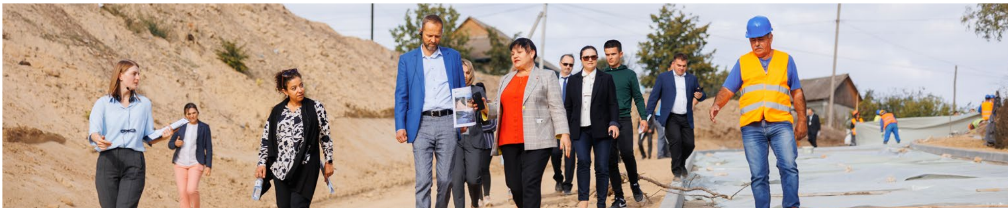
European Union Ambassador, Jānis Mažeiks, and UNDP Resident Representative to the Republic of Moldova, Dima Al-Khatib, visiting the construction site in Slobozia Mare, Cahul district, 21 September 2022.
